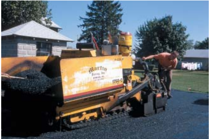
Martin Paving replaces its pavers every eight years — after five years on the front line and three years as a backup machine.
