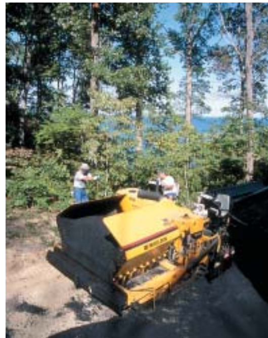
Contractors say the the paver's conveyor and auger system ease paving up and down hills.
